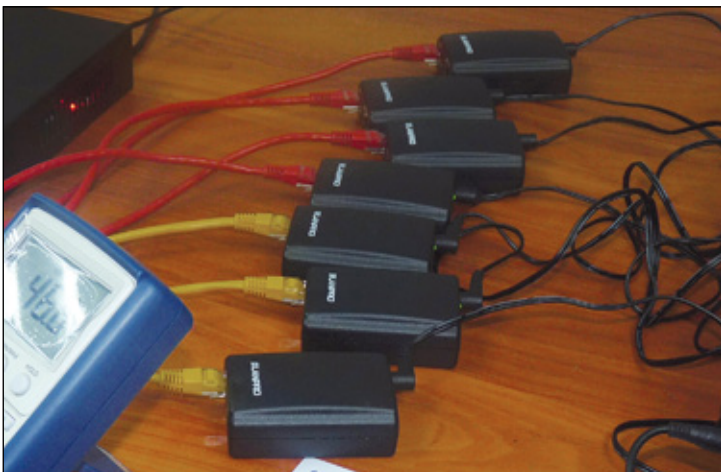
Figure 12. PoE Splitters loading the switch
